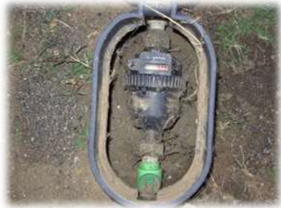
Domestic metered connection
