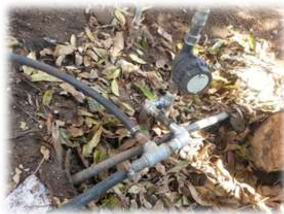
Unauthorised water connections
